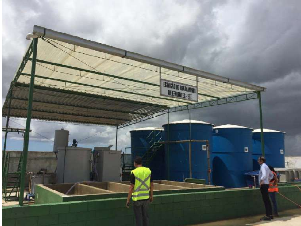
Treatment Effluent Station
